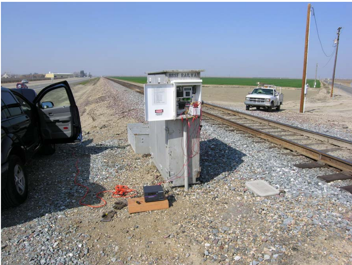
Figure 14: The heavy-duty DC supply rests on the board in the foreground. It is powered via the orange extension cord that comes from the inverter. Alligator clip leads were used to make the remaining connections. The new controller rests near the lower right-hand corner of the open white control box.
